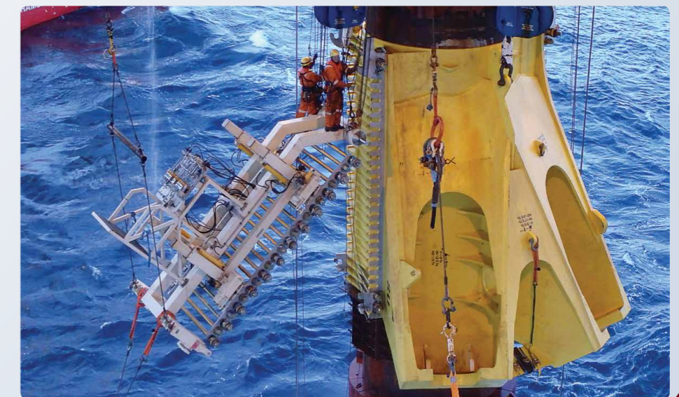
Installation of the 150Te clamps to the platform legs required the design and fabrication of hydraulically operated bolt racks, to make the task safer and more efficient for the rigging crew
